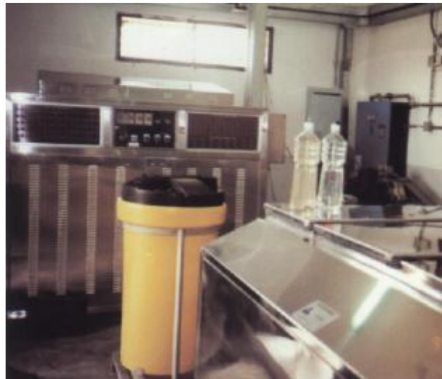
UV/Ozone system installed at Fairview Park, capacity 250,000LPH. Bottles indicating before and after passing the system
